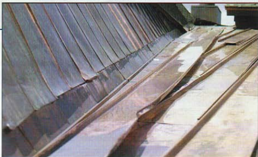
SNOW PILED HIGH IN ASPEN. BELOW, ROOF DAMAGE CAUSED BY ICE DAMS.
